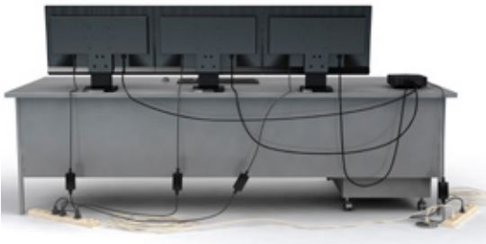
Before Messy cables.
